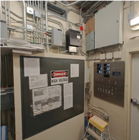
Fire control system
