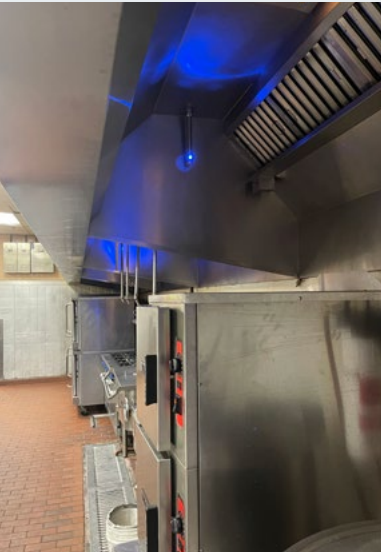
ECOAZUR installed at Hilton Salt Lake City Center
