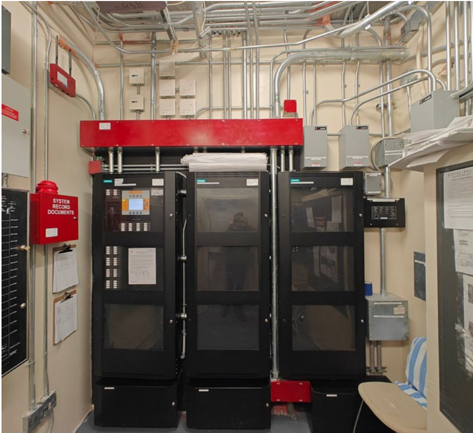
Fire control safety system
