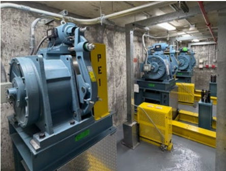
Raised elevator equipment
