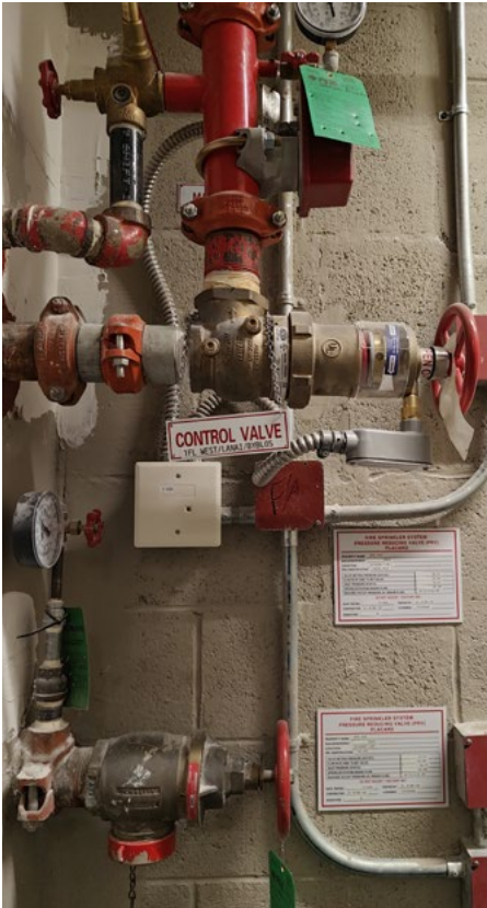
New sprinkler system installed
